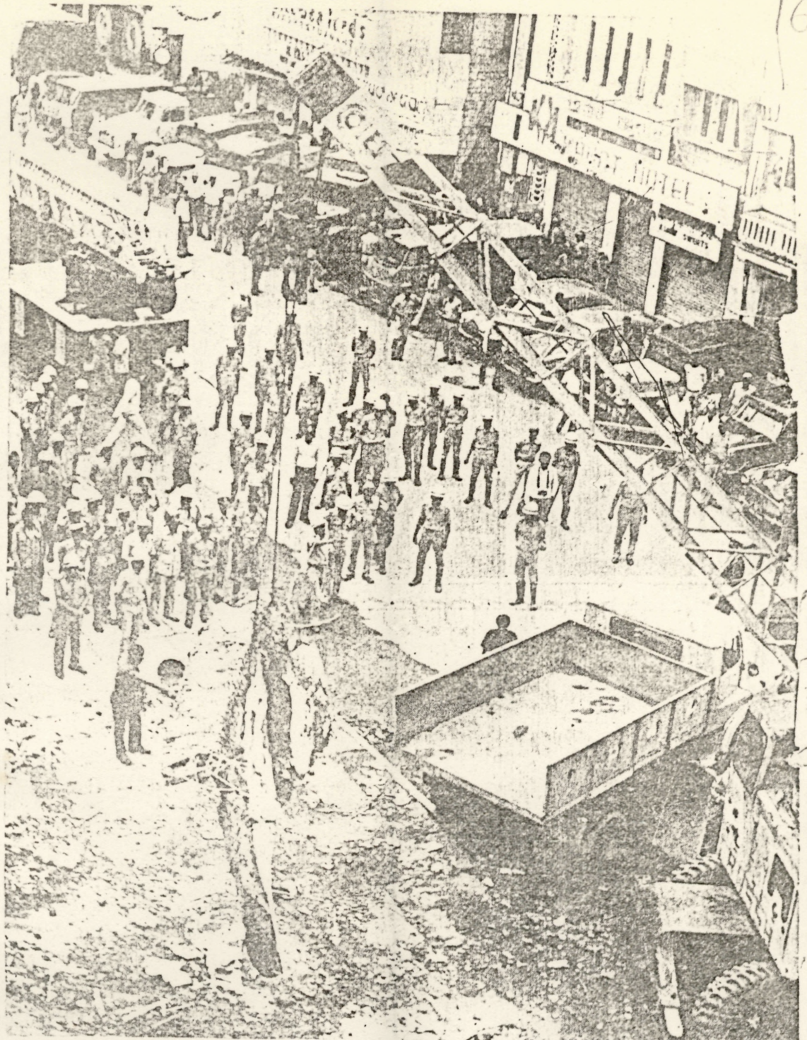
A massive slab of concrete being lifted out of the debris with the help of a crane.
