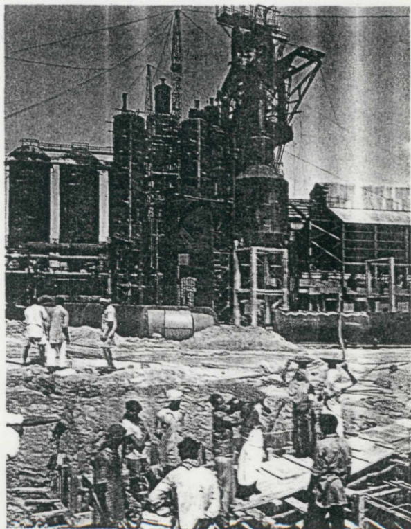
THESE WORKERS are building a new India. . . . The works are designed to produce 800,000 tons of finished steel products a year.
