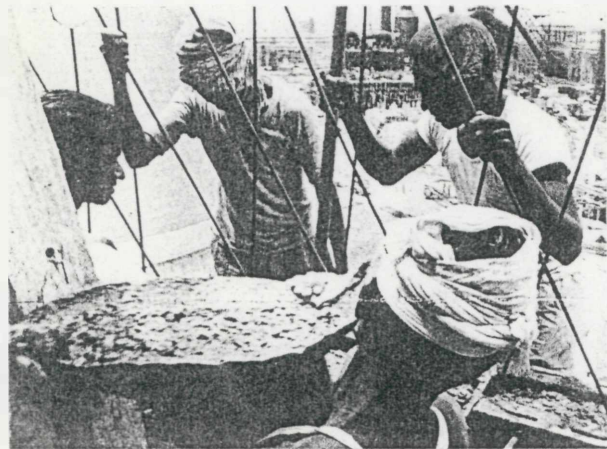
BUILDING the reinforced concrete wall of a cooling tower, one of many jobs that are being tackled by Indians.
